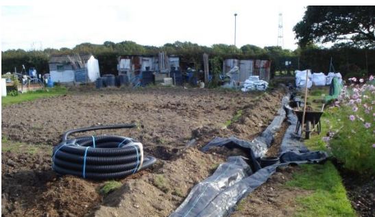
Installing the perforated land drain, well it would be, but we've all gone to tea!
